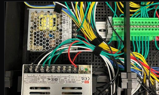
DAQ AND POWER WIRING
