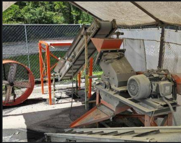
THE CRUSHING AND SCREENING LINE
